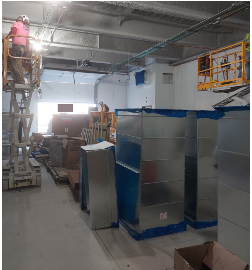
Fig. 2. It's important to make plans on where you want material delivered to avoid situations like a backed-up loading dock.
